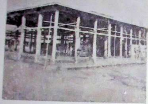
The Guru Nanak Auditorium under construction. When completed it will fulfil a long-felt need of the students. It is proposed to house the Reading Room and some Department I Rooms on the upper storey of this Auditorium.
